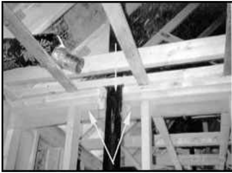
Joist cut - An example of an over anxious plumber with a chainsaw who has now jeopardized the structural integrity of the framing to allow for a bathroom vent stack.
