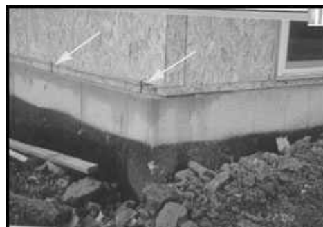
Anchor Bolts - Anchor Bolts are supposed to go on the inside of the house to secure it to the foundation!
