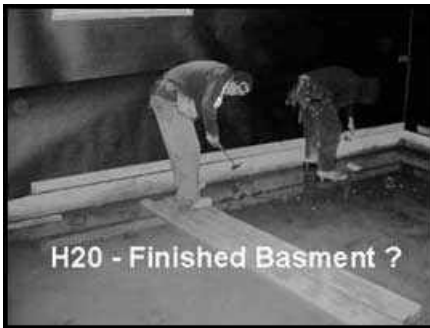
H2O Basement - these workers are actually standing in about 2 inches of water while they are attempting to finish the basement framing. Note all the black mould growing on the back wall just above the water line!!
