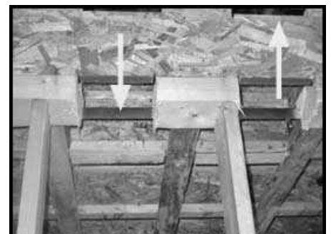
Framing Cut - Here is an example of what can happen to a properly framed (and municipally approved) new home after the heating contractor went chainsaw crazy. .
