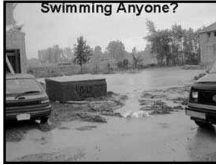
Water logged - This residential building site looks more like a good place for a quick dip on a hot summer day!
