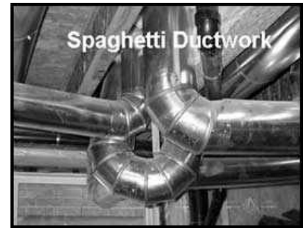
Spaghetti Ductwork - What this Home Inspector likes to refer to as Spaghetti Ductwork! - It bends and curls. Looks impressive, but wouldn't want to be paying the heating bills.
