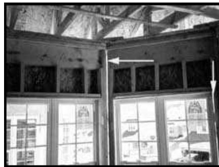
Framing Gaps - When this homeowner asked for air conditioning, we don't think this is quite what he had in mind!
